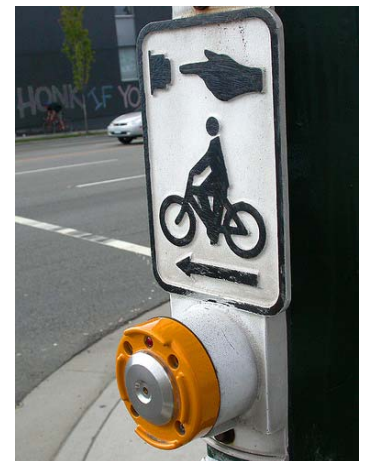
A CYCLIST PUSH BUTTON ALLOWS BICYCLISTS TO ACTIVATE TRAFFIC SIGNALS WITHOUT DISMOUNTING THEIR BICYCLE.
